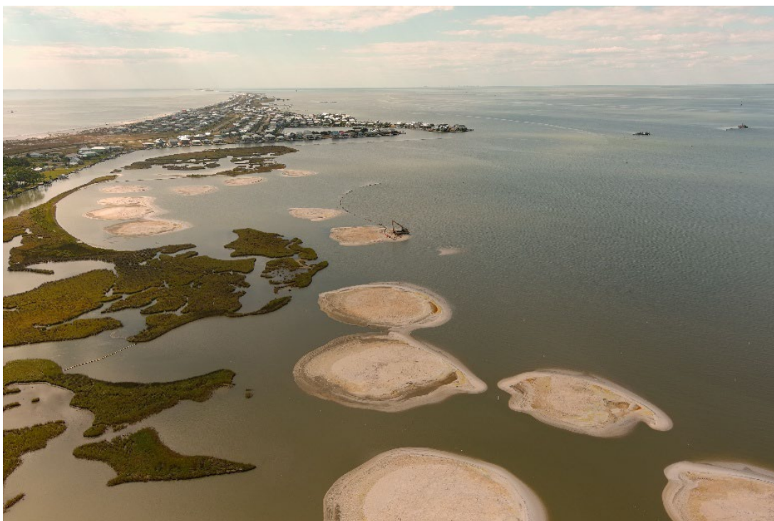
The new marsh mounds in Graveline Bay, while under construction. Photo courtesy of Moffatt & Nichol.
