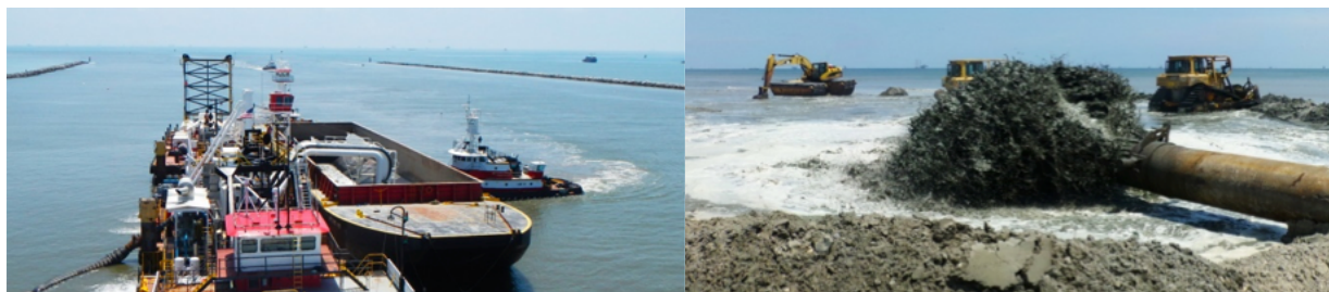
Figure 18. An example of double handling utilized for the Caminada Headlands Restoration project. The left picture illustrates a secondary dredge, in this case a CSD, pumping out of a barge filled with offshore material dredge by a primary vessel. The right picture shows a terminal section of the pump to shore pipeline and ancillary sculpting equipment actively moving dredged sediment (Source: CEC, 2012).
