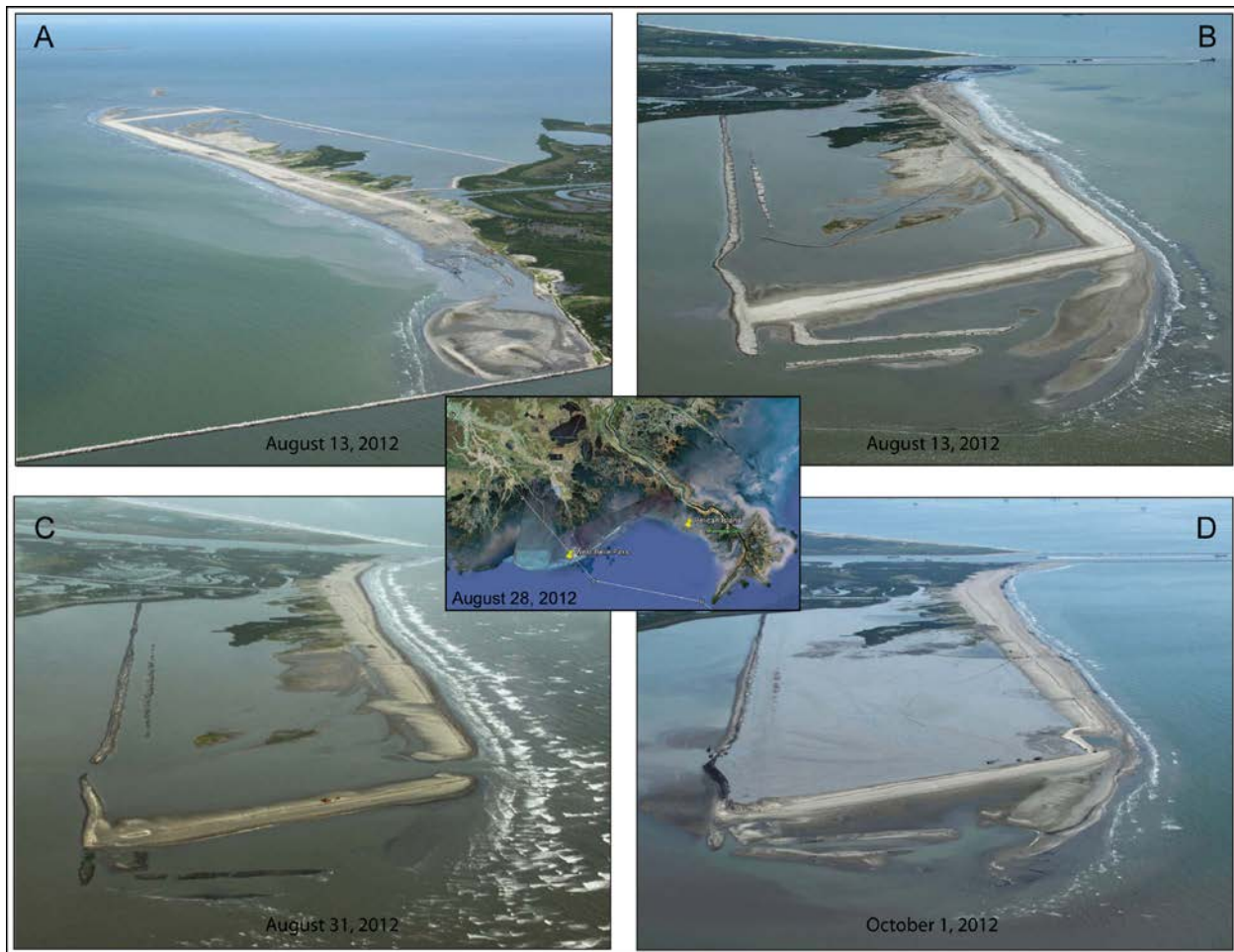
Figure 9: CPRA Restoration Project TE-52 performed on West Belle Pass Barrier, four photos show the containment dike and sediment nourishment progress. A) Aerial view from the east of project under construction on August 13, 2012. The west Belle Pass jetty is in the foreground B) Aerial view from the west of project under Construction on August 13, 2012. A recurved spit formed from longshore transport processes. C) Aerial view from the west of project area on August 31, 2012, after Hurricane Isaac passed directly over the barrier resulted in storm induced breach in containment dike and overwash of 104 yds 3 of sand. D) Aerial view from the west of project October 1, 2012 after sheetpile closure of containment dike breach. Google Earth imagery (center) shows Hurricane track over the project area on August 28, 2012. (Photographs are courtesy of Weeks Marine & Aerophoto for NOAA Fisheries; Parker et al., 2012).
