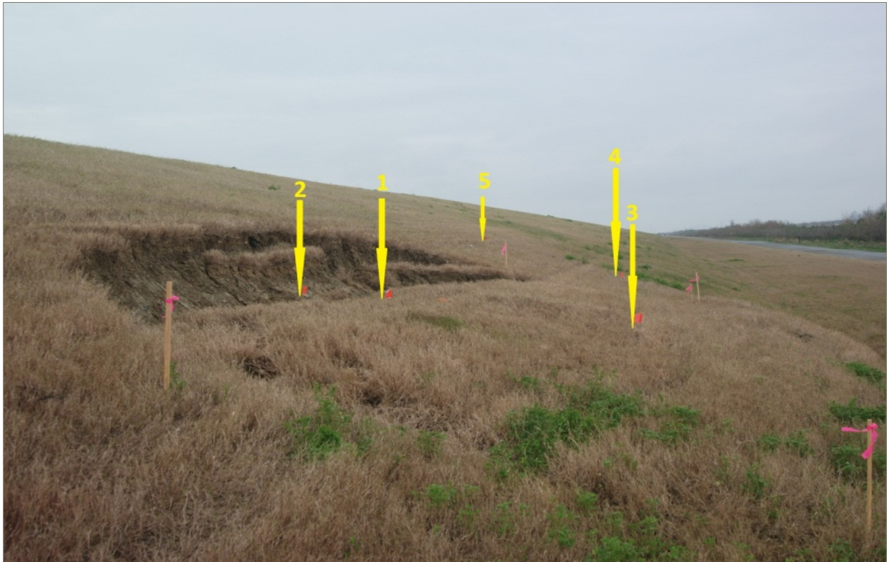
Figure 5. Shallow slope failure near toe of earthen levee for New Orleans east back segment. Numbered arrows indicate sampling locations for a previous study. (Provided by R. Brouillette, CPRA).
