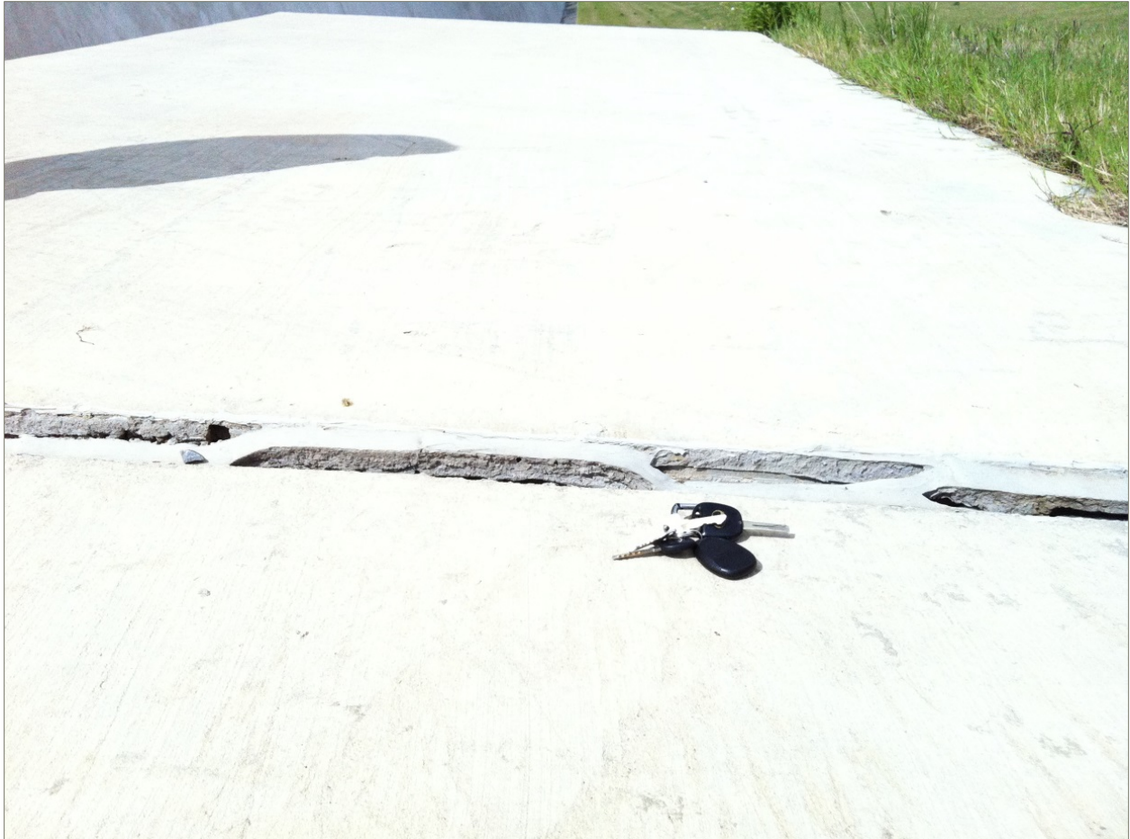
Figure 4. Differential settlement at transition between T-Wall for Lake Borgne Closure (background) and earthen Levee for New Orleans east back segment (foreground) - Taken by R. Gilbert on July 16, 2013.
