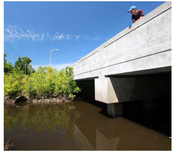
Bees Ferry Road One of the significant bottlenecks in the Creek's drainage.
