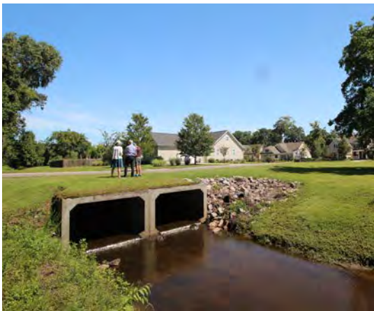
Upper Church Creek Development Development along the upper portion of the creek constricts it's flow.
