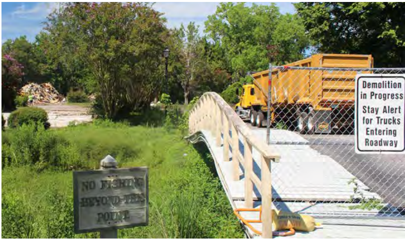
Shadowmoss Buyout Properties Recently, homes within the floodplain were purchased and demolished by FEMA.
